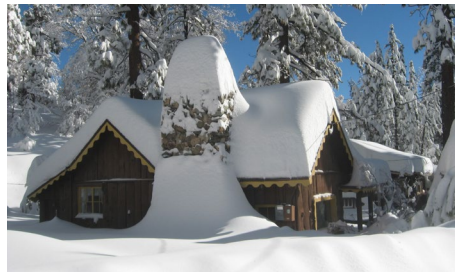
Heavy snow and ice damming can weigh down your roof potentially causing water leaks or worse.
