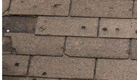
Large and fast-moving hail may compromise your roof structure's integrity.
